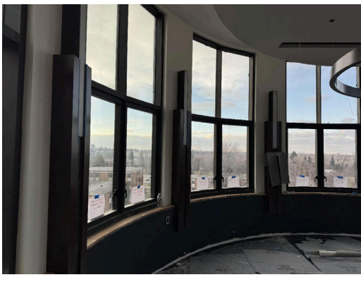
2nd Floor: Walls have been sanded and received their first coat of paint. This allows follow-on trades to begin installing finishes like trim, fixtures and casework.
