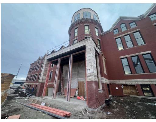
North Entry: Stonework is complete, and a final cleaning will remove grout haze and bring out the full color and detail of the stone.
