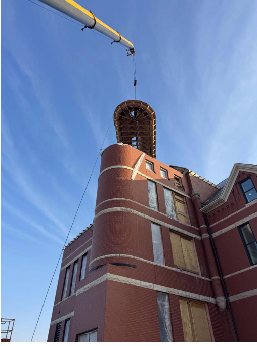
Exterior – West Roof: Staircase system roof constructed at ground level and crane-set into place.
