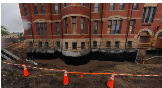
Foundation repairs are complete. New waterproofing system has been sprayed on 7' until backfilling catches up.
