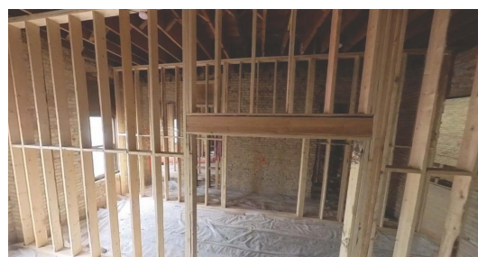
Temporary shoring walls were installed to remove the old steel structure and install a new one.
